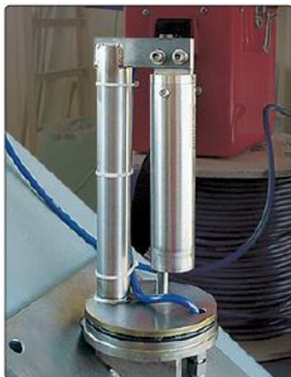
• Model 6350 installation using a custom mounting bracket designed for concrete face rock fill dam applications (shown with protective cover removed).
